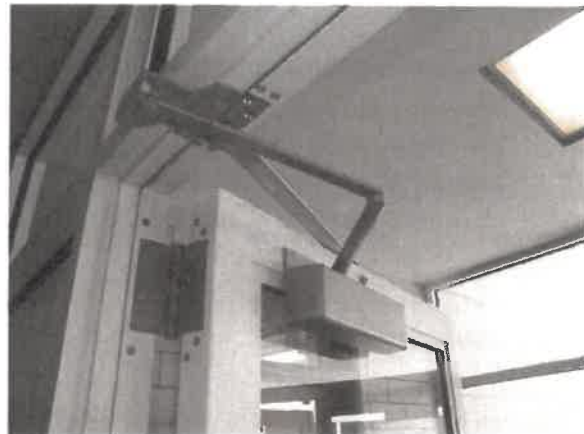
Figure 20: Original (ca. 1993) and supplemental overhead door closers/stops.
