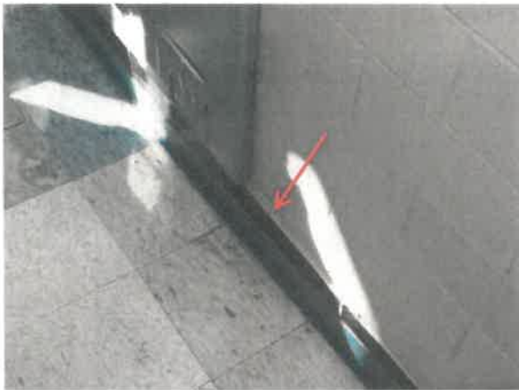
Figure 49: 1956 masonry wall construction displaced by the force of water and silt from 2014 flood event.
