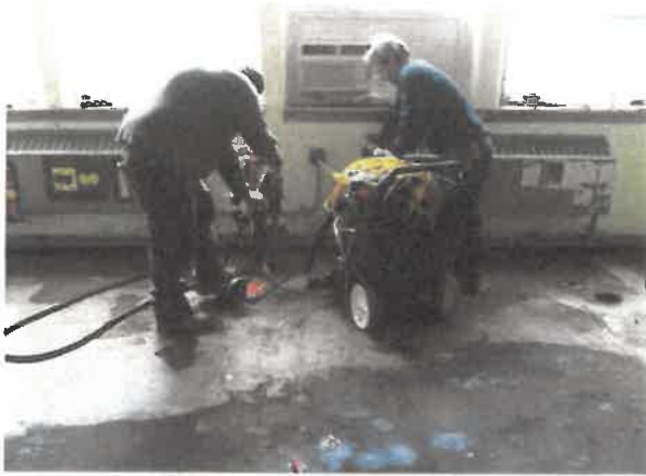
Slab Jacking at Health Office at Spring 2014 Due to hydrant line burst under the building.
