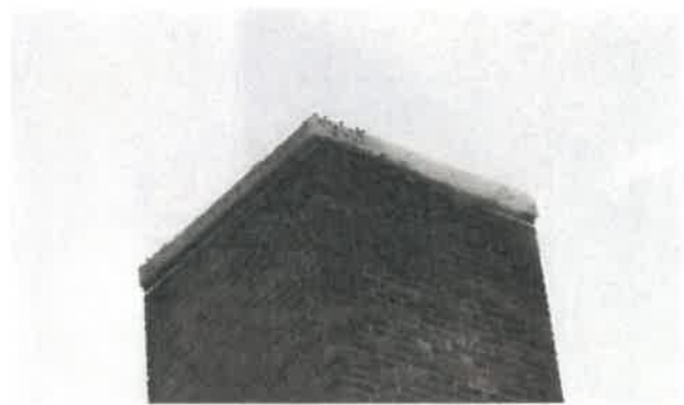
Boiler Room Chimney Note efflorescence and some loss of mortar at joint.
