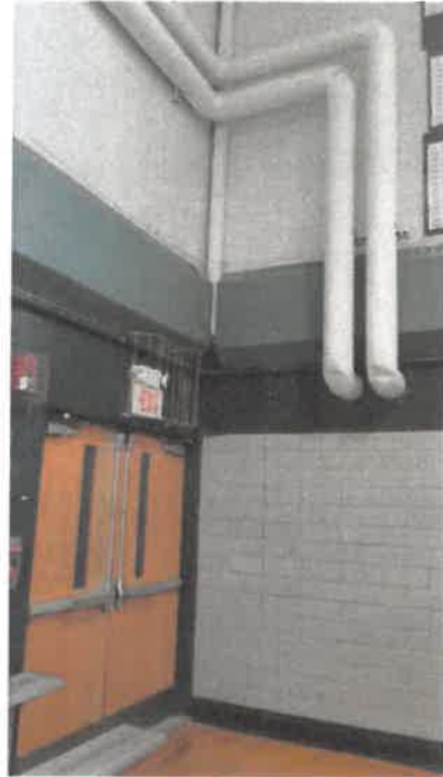
Vertical Crack at NW Gymnasium Corner
