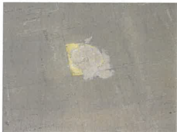
Figure 48: Damaged and patched vinyl asbestos floor tiles.
