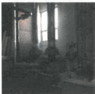
Gas Fired Hot Water Heaters
