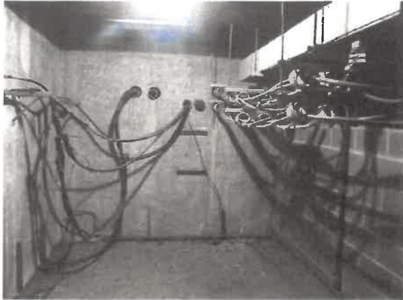
Figure 60: Existing primary electrical service in Apparatus Room utility vault.
