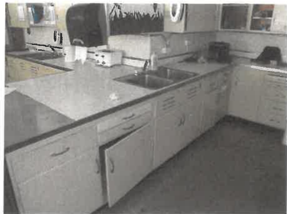
Figure 43: 1950s era home economics kitchen cabinets and counters.
