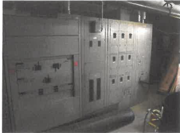
Figure 61: Original 1956 main switchboard (right) and added 1993 switchboard in Apparatus Room.
