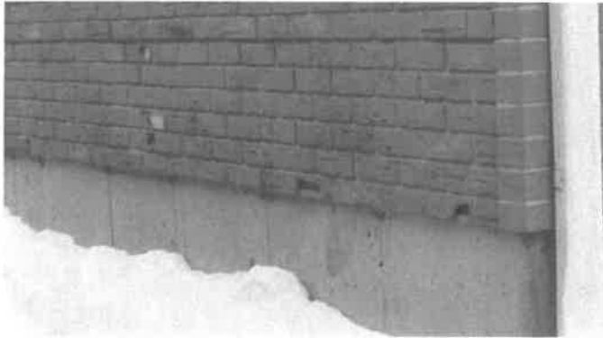
Cafeteria Addition Note impact damage on "faux brick" plastic façade
