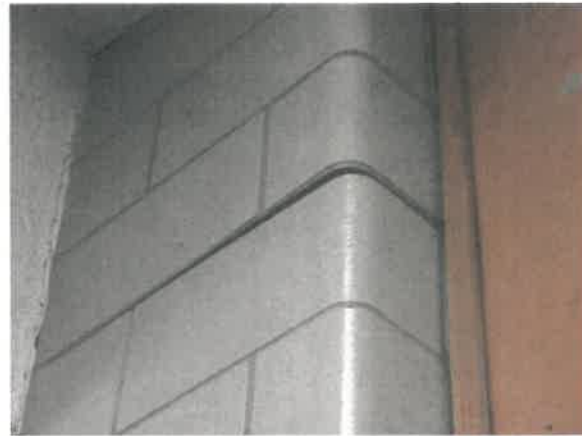
Figure 50: Stress release crack at 1956 auditorium.
