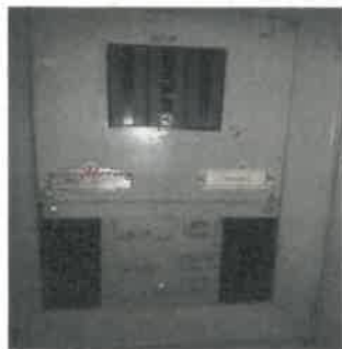
Frank Adam Panelboard
