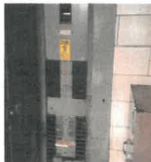
Gym I-T-E Panelboard
