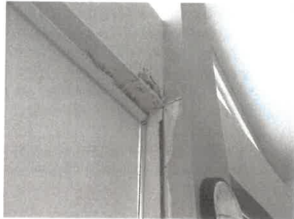
Figure 13: Damaged interior finishes at 1993 media center.
