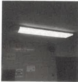
Typical Hallway Light
