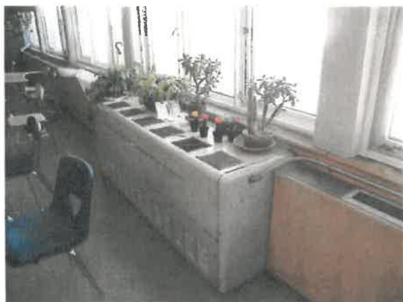
Figure 55: Original unit ventilator in 1956 classroom.
