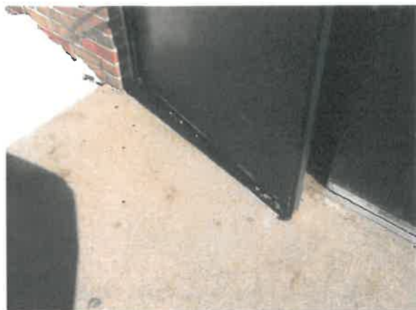
Figure 21: Damaged egress door from 1993 gymnasium.
