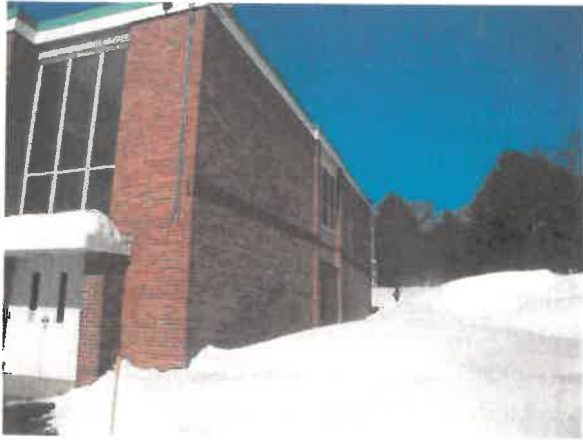
Figure 07: East end of the 1956 “Junior wing” where modular classrooms were removed in 2014.
