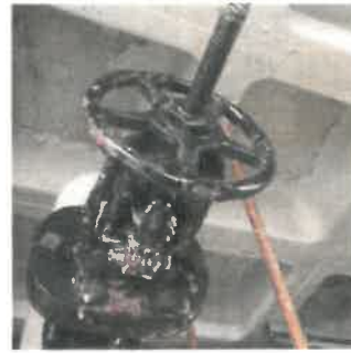
Apparatus Rm – Corroded Gate Valve
