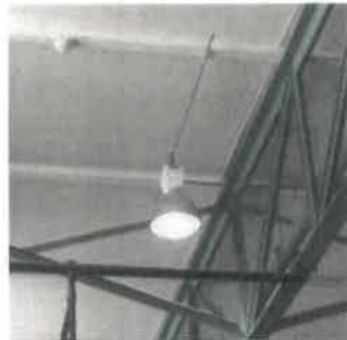
Gym Smoke Detector
