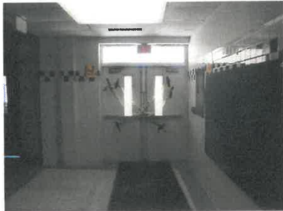
Figure 11: Caution tape at 1993 egress doors below icicles.
