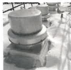
Rooftop Exhaust Fans
