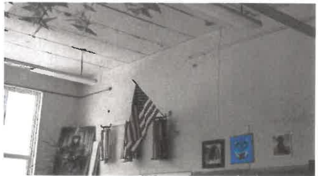
Masonry Vertical Crack at Metal Shop
