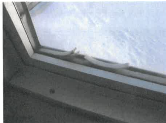
Figure 17: Deteriorated gaskets at aluminum windows.
