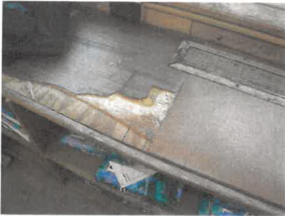
Figure 42: Damaged countertop surfaces at 1956 classroom shelving units.
