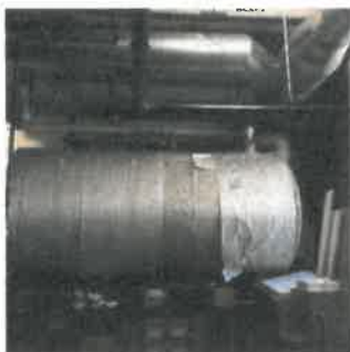
Domestic Hot Water Tank #1
