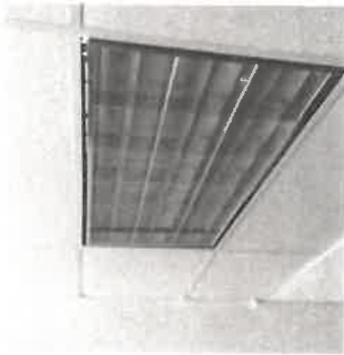
Typical 1993 Addition Lights
