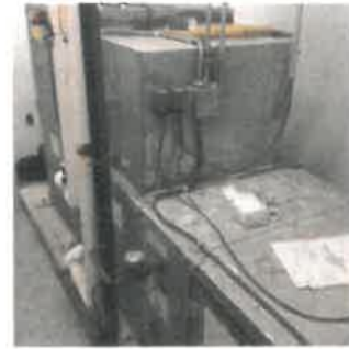
Air Handling Unit AH-1
