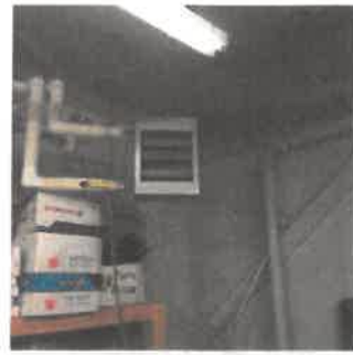
Hot Water Unit Heater
