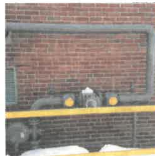
Natural Gas Service
