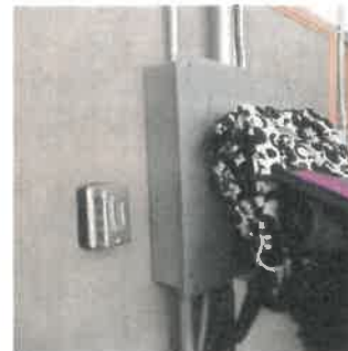
Typical Classroom Panelboard
