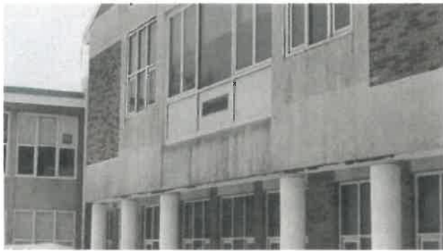
Library Façade at Courtyard Note corrosion along its edges
