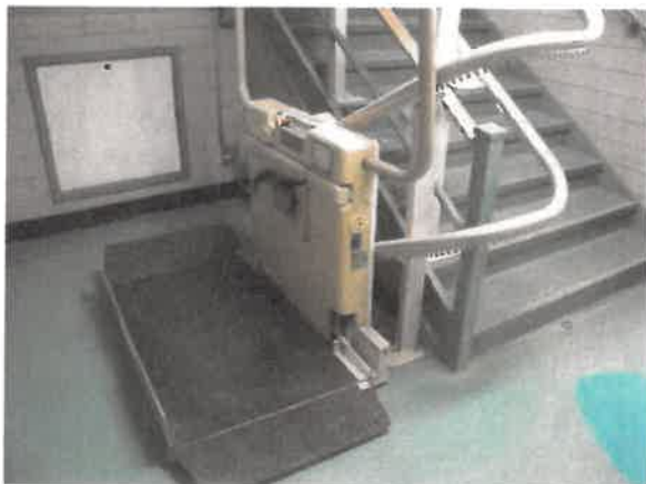
Figure 39: Inoperable stair lift at 1956 "Junior wing."
