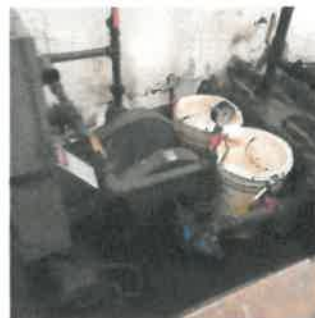
Fuel Oil Supply Pumps
