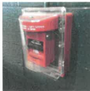
Typical Gym Pull Station
