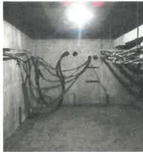
Primary Cable Vault
