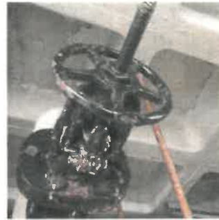
Apparatus Rm – Corroded Gate Valve
