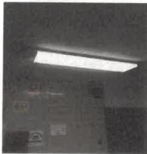
Typical Hallway Light
