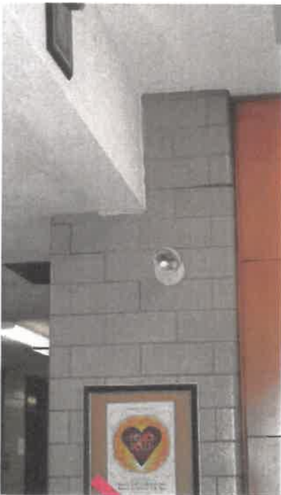
Step Cracking at Glazed Tile Pilaster Corner of Auditorium
