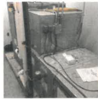
Air Handling Unit AH-1
