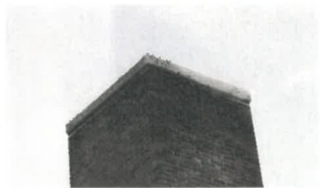
Boiler Room Chimney Note efflorescence and some loss of mortar at joint.
