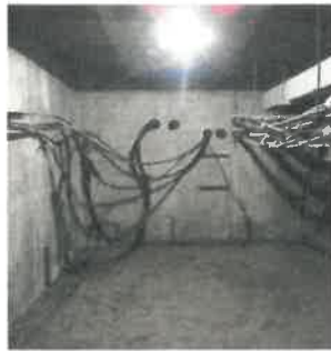
Primary Cable Vault
