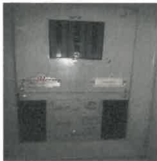
Frank Adam Panelboard
