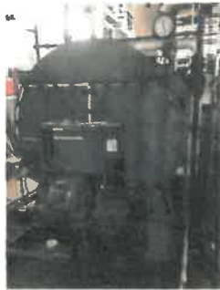
Fire-Tube Steam Boiler
