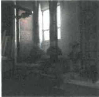
Gas Fired Hot Water Heaters
