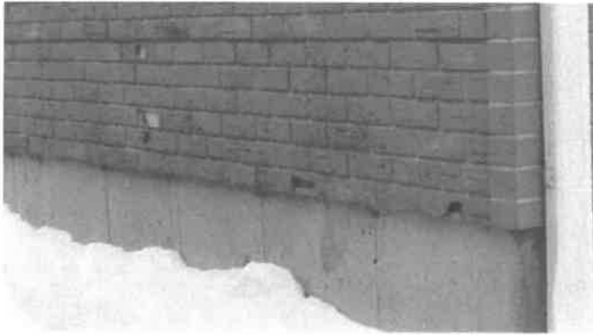
Cafeteria Addition Note impact damage on "faux brick" plastic façade
