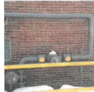
Natural Gas Service
