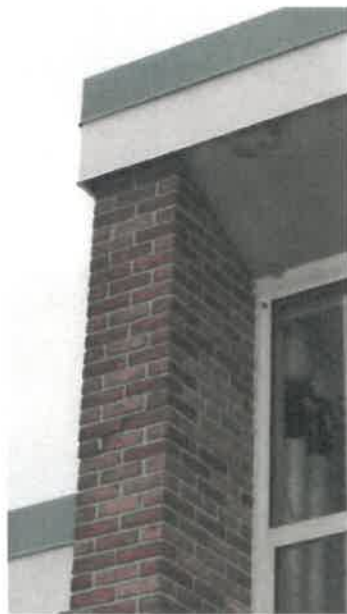
Blade Wall adjacent to Door A3 Note step crack at window mid-height
