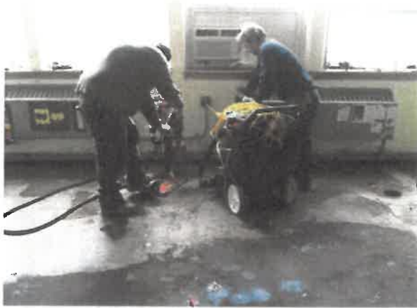
Slab Jacking at Health Office at Spring 2014 Due to hydrant line burst under the building.
