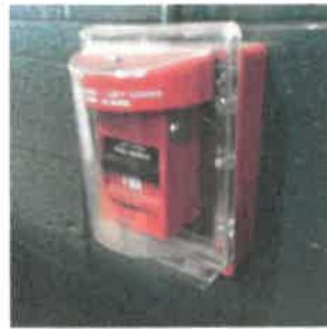
Typical Gym Pull Station
