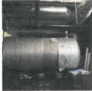
Domestic Hot Water Tank #1
