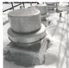
Rooftop Exhaust Fans
