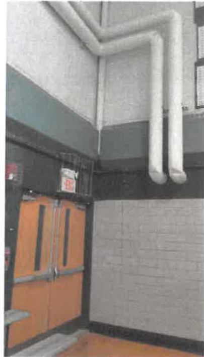
Vertical Crack at NW Gymnasium Corner
