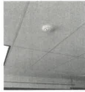
Typical Smoke Detector
