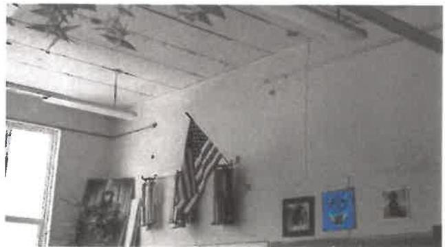
Masonry Vertical Crack at Metal Shop
