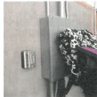
Typical Classroom Panelboard
