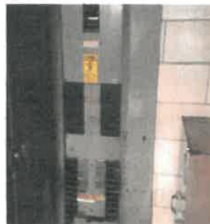
Gym I-T-E Panelboard
