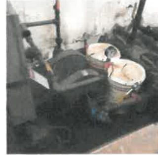
Fuel Oil Supply Pumps
